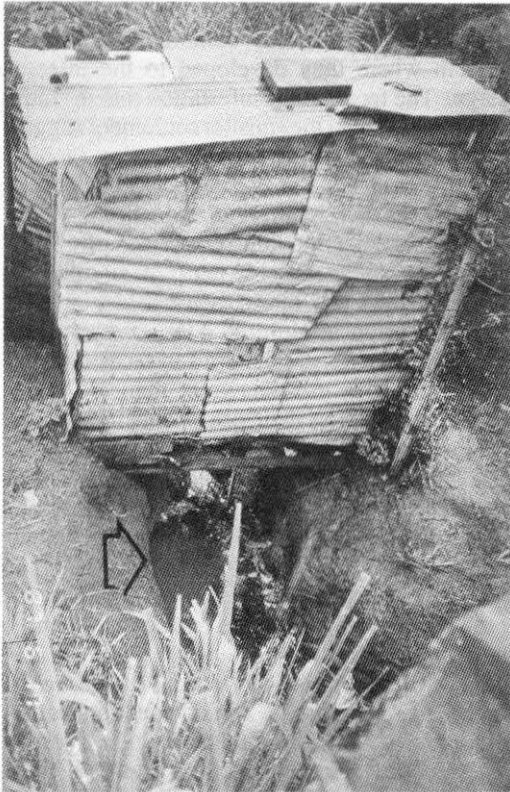
Fig. 1. Typical latrine from the squatter settlement. The gutter (arrow) with raw sewage and the feces circulate throughout the community.
